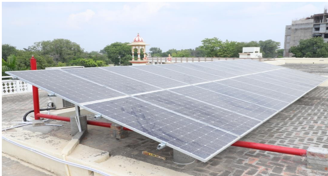
Solar panel 45KW
