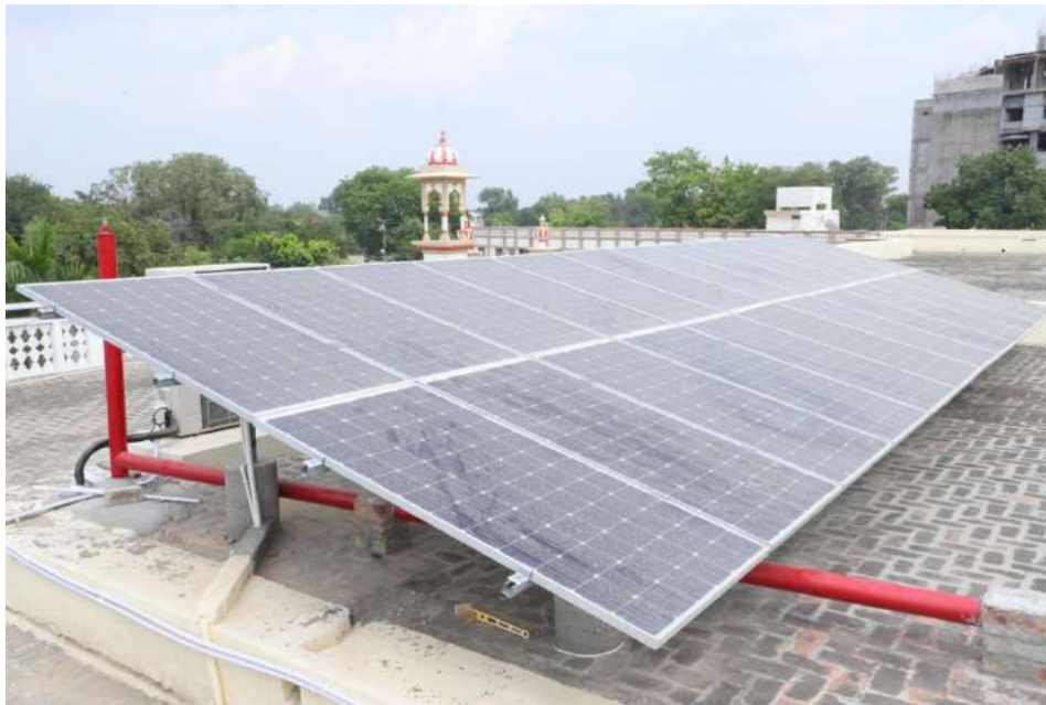
Solar panel 45KW
